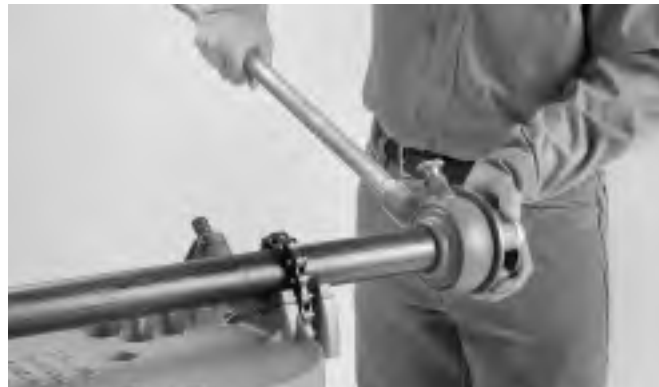
Figure 3 – Sliding Threader On Pipe
